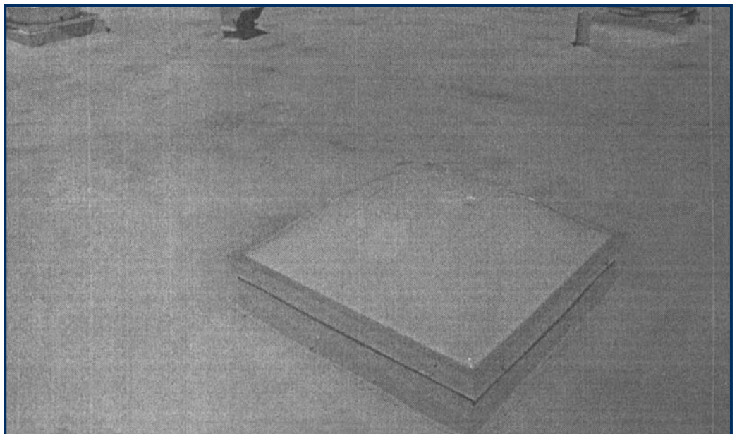
The skylight has been damaged by hail, but the SPF roof exhibits no visible signs of damage.
