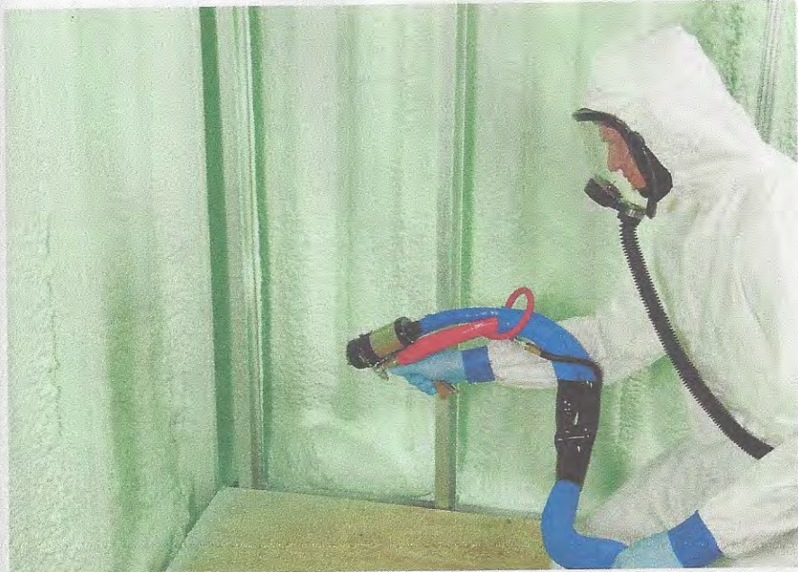
Quality foam requires the correct combination of heat, pressure and spray gun configuration. Photo courtesy of Demilec.
