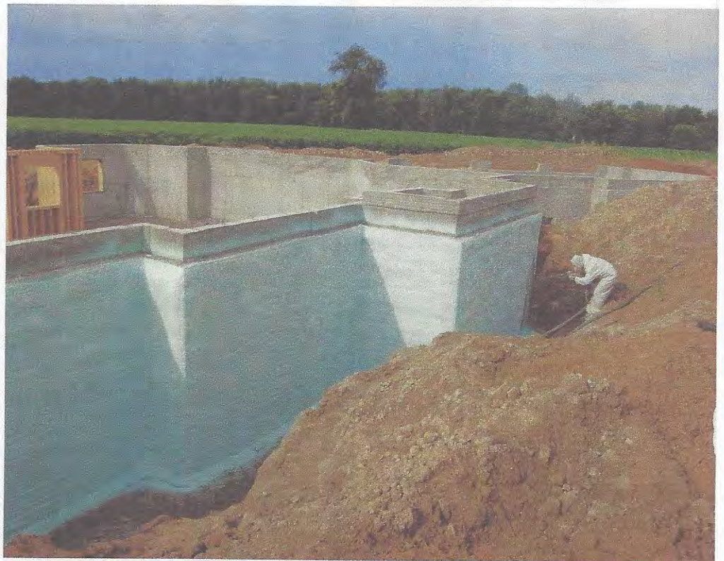
Foam that is hard to remove and leaves bits of foam on the substrate is considered the best adhered. Here, SPF insulates a residential basement. Photo courtesy of Demilec.
