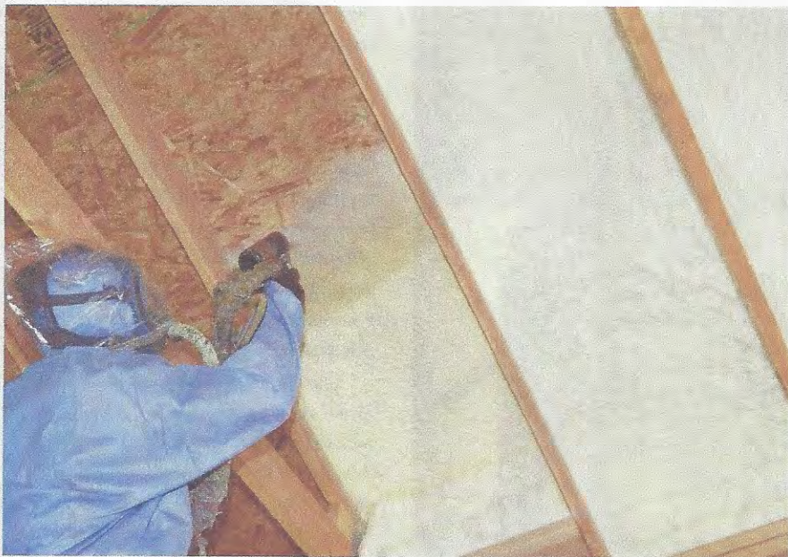
Open-cell SPF is typically installed in one lift to a stud wall or ceiling cavity to full thickness. Start at the bottom and work up. Photo courtesy of Demilec.
