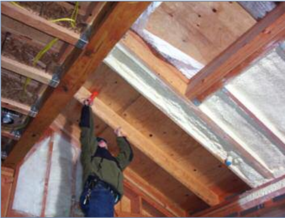
Photo 7 – Measure moisture content of the substrate before installing the foam. Wood substrates such as plywood and OSB should contain no more than 18% moisture as measured by a Delmhorst Moisture Probe (or equivalent measuring tool).
