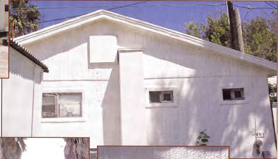
Figure 14 – Same building after Hurricane Dolly in 2009.
