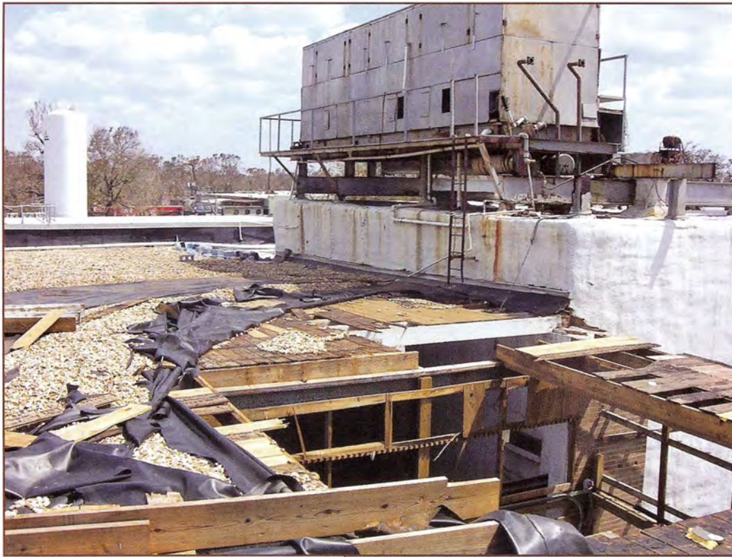
Figure 9 – Internal pressurization during Hurricane Katrina destroyed a tongue-and-groove wood deck at this ice plant.
